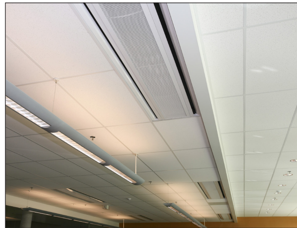
CBAL-24 installed in the ceiling of a school
